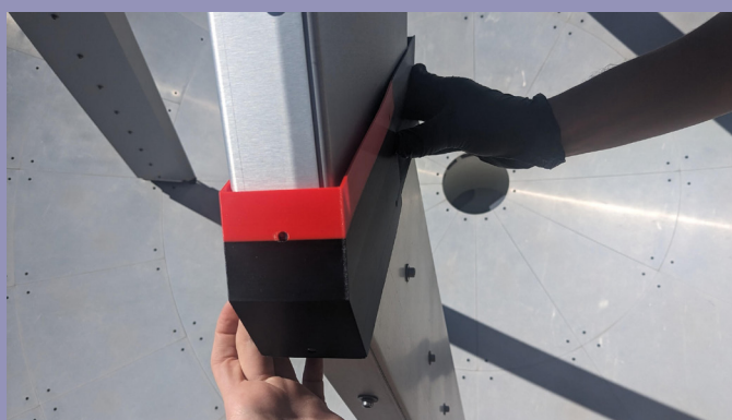
Figure 1: On the summit of Maunakea, CE engineer Abigail Unger performs test fittings of 3D-printed models of the new shielding components. These test fits were successful in verifying dimensional requirements, and came at the conclusion of a multi-year engineering study centered on readying the SMA for solar observing.
